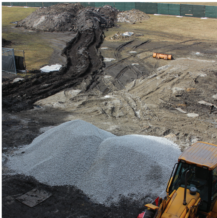
The construction site on the north athletic fields outside of the ACT testing rooms where students were disturbed on Mar. 3 | Merrill
