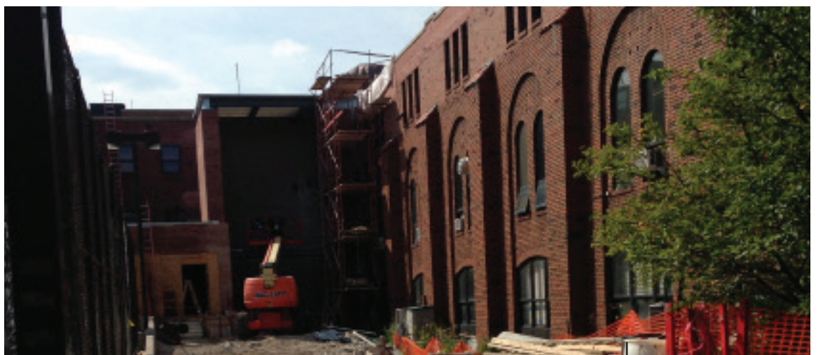
New elevator construction during the ADA renovation process, near field house entrance | Minturn
