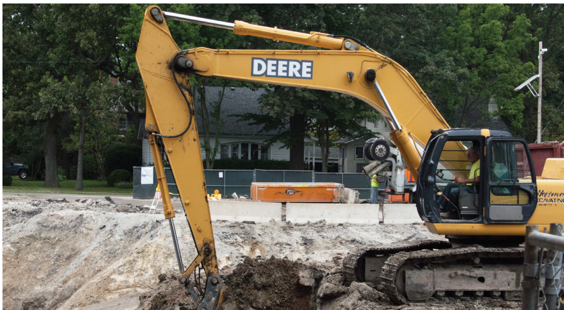
Construction crews continue to make progress on the renovation as students and teachers return | Lutschaunig
