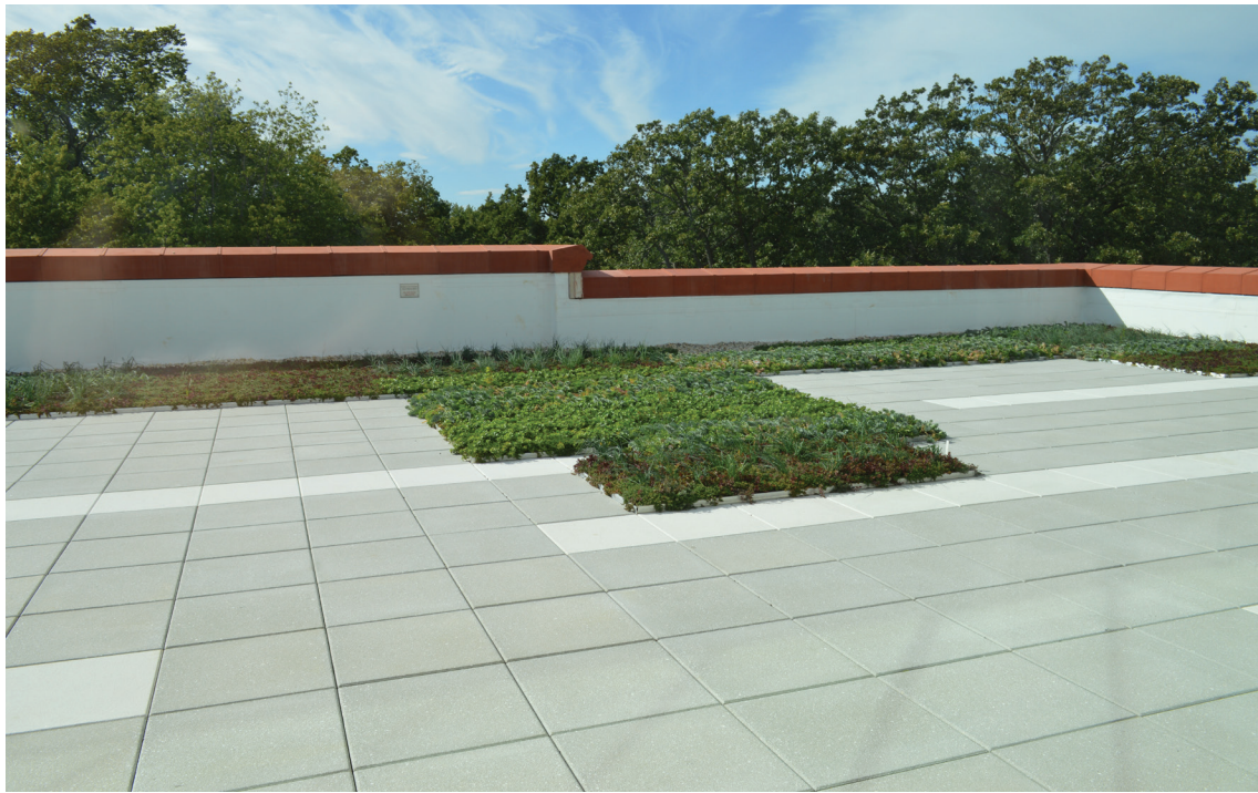
New roof deck offers a supervised outdoor area for students to meet with friends and eat in the fresh air | Zervas
