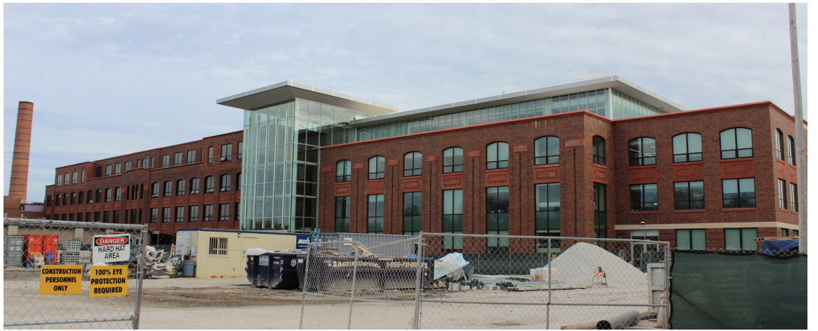
Phase two of construction is set to be completed by the beginning of the 2017-2018 school year in Sept. | Josellis
